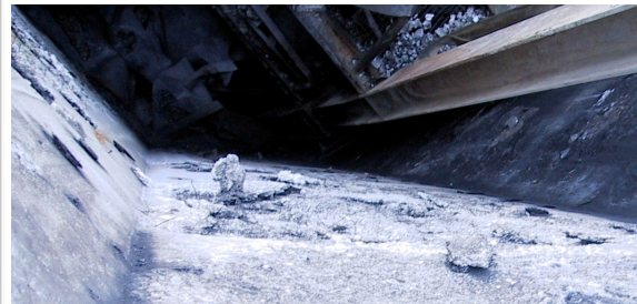
Fig. 11 Detail of damaged concrete containment
